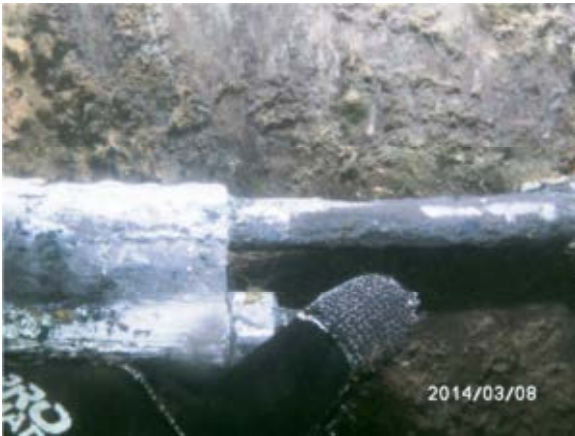
Photo 21A – Stripped / corroded connector
