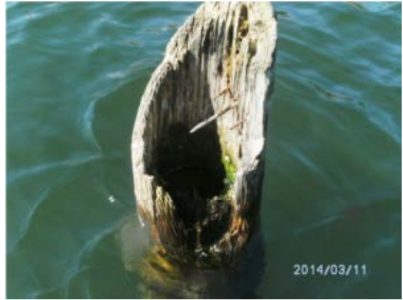
Photo 26A – Deteriorated mooring pile
