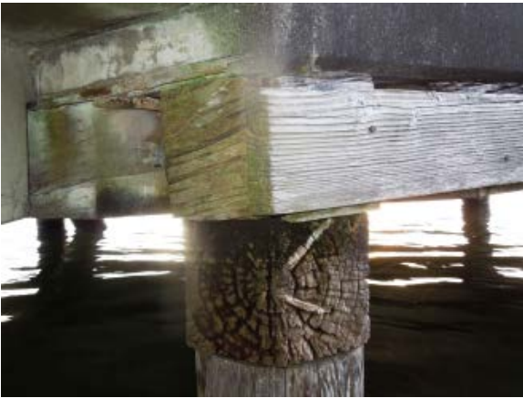
Photo 25A – Deteriorated cap beam (small pier)
