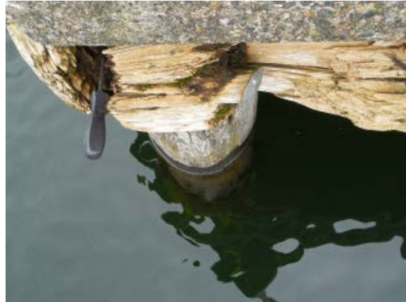
Photo 14A – Deteriorated cap beam
