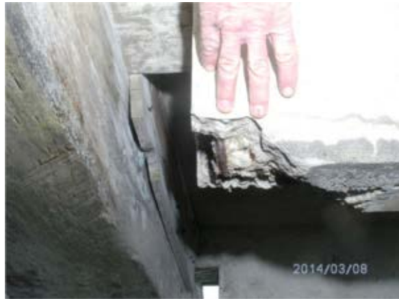
Photo 16A – Spalling at underside of precast "T"
