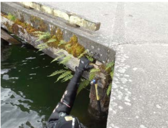
Photo 11A – Moss / vegetation at pier edge
