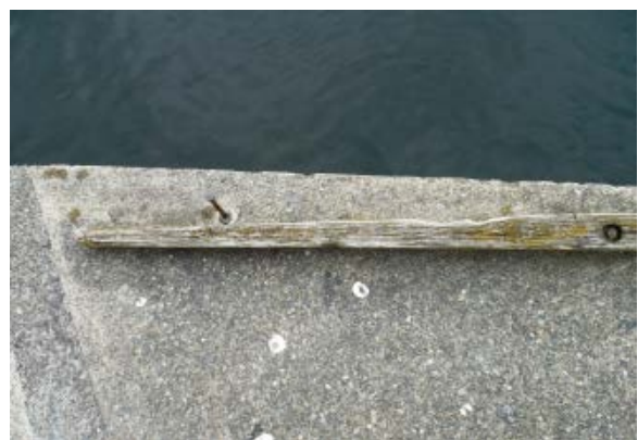
Photo 12A – Deteriorated / loose bull rail
