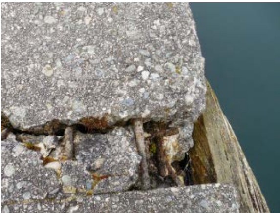
Photo 9A – Deteriorated pier slab
