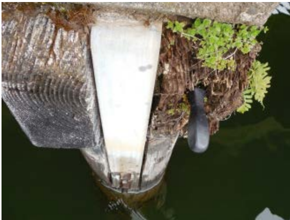
Photo 15A – Deteriorated cap beam end
