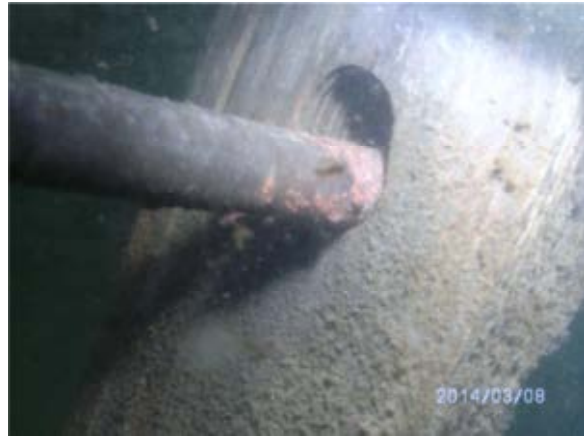
Photo 20A – Loose connector at substructure
