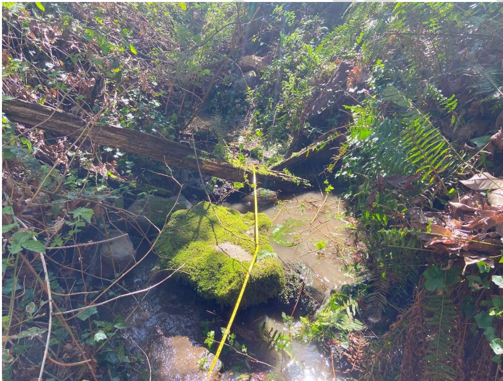
Photo 2.3 View of watercourse looking upstream about 50 feet downstream of the SE 65 th Street culvert outlet (STA 2+20). Note, flanking of rock check dam and displacement of rock.
