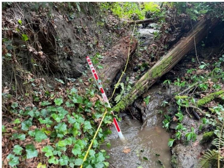
Photo 2.1 View of watercourse looking upstream from the base on the knickpoint (STA 3+50). Note, level rod indicating relative drop in bed elevation.
