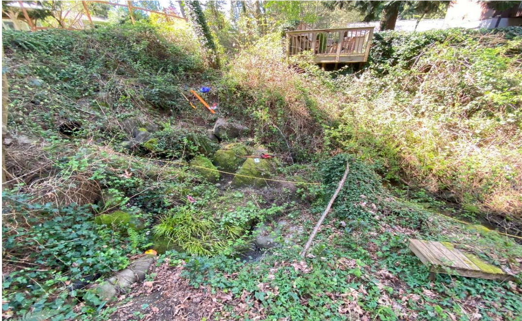
Photo 2.4 View of watercourse standing on right bank facing west about 30 feet downstream of SE 65 th Street culvert outlet (STA 2+00). Note, observed left bank erosion and displacement of outlet protection rock.
