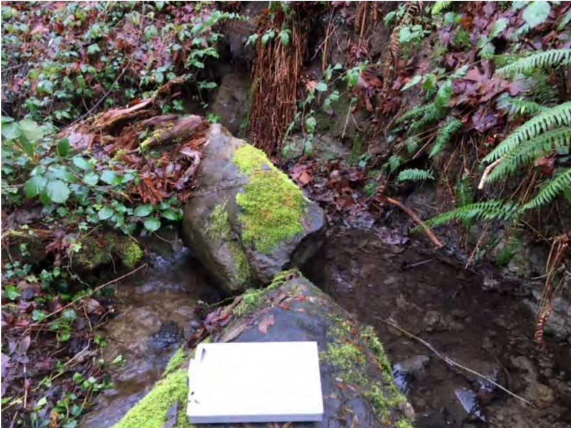
Bank erosion below pipe outfall from 8010/8020 SE 65 th Street. 01/19/2018
