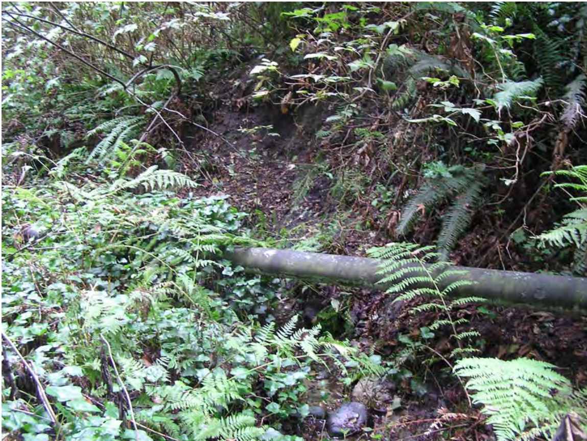
Looking Downstream at Exposed Sewer Pipe 9/12/2005
