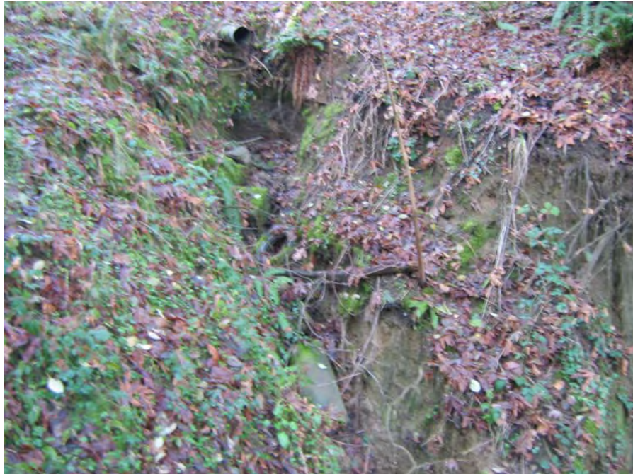
Looking Upstream at Upper Half of Erosion Problem 12/14/2005
