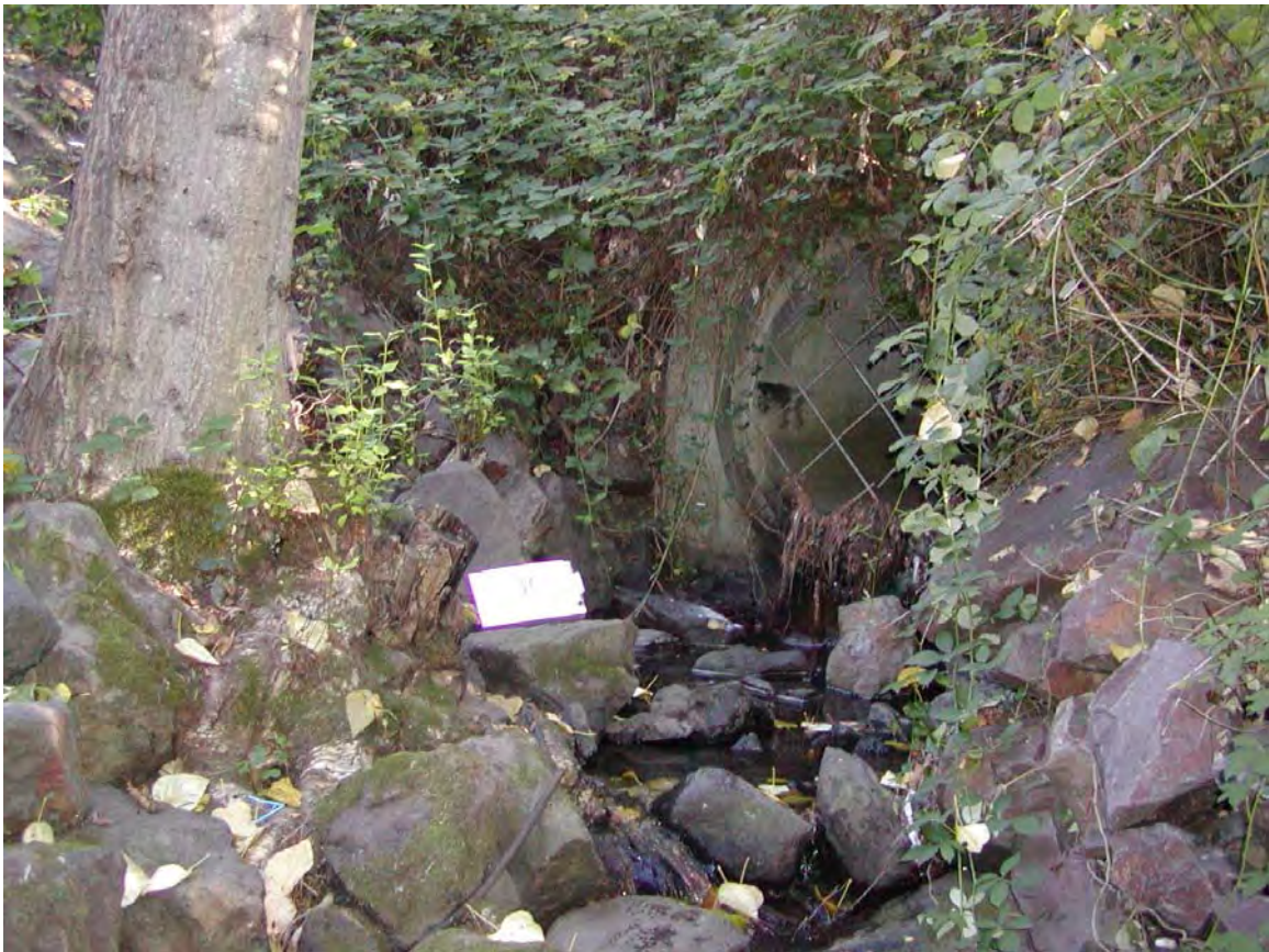
Looking Upstream at 60" Outlet 9/24/2005
