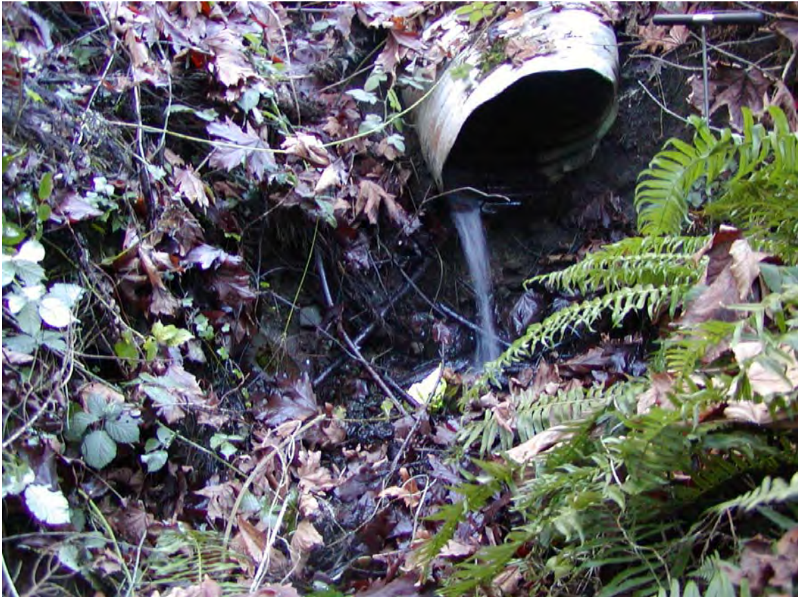
Erosion at Pipe Outlet (pipe crushed) 12/8/2005
