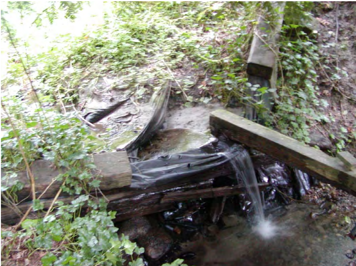
Looking Upstream at Failing Timber Dam 9/28/2006
