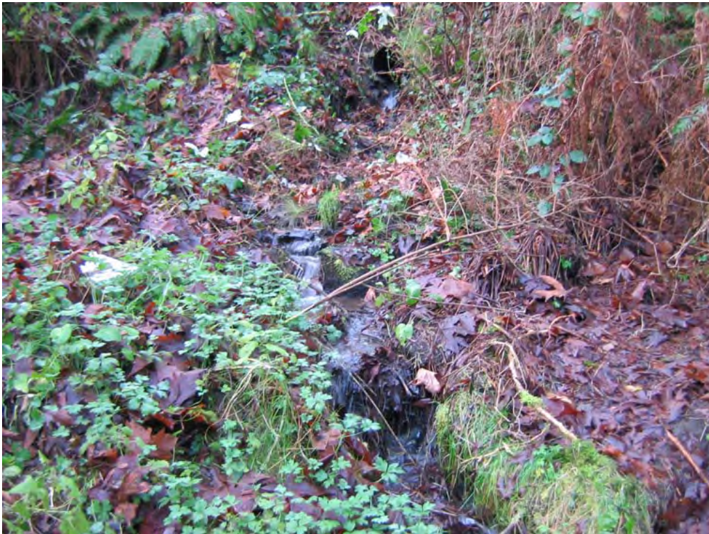
Looking Upstream at Steep Channel and Outlet. Erosion of Bank on Left. 12/14/2005
