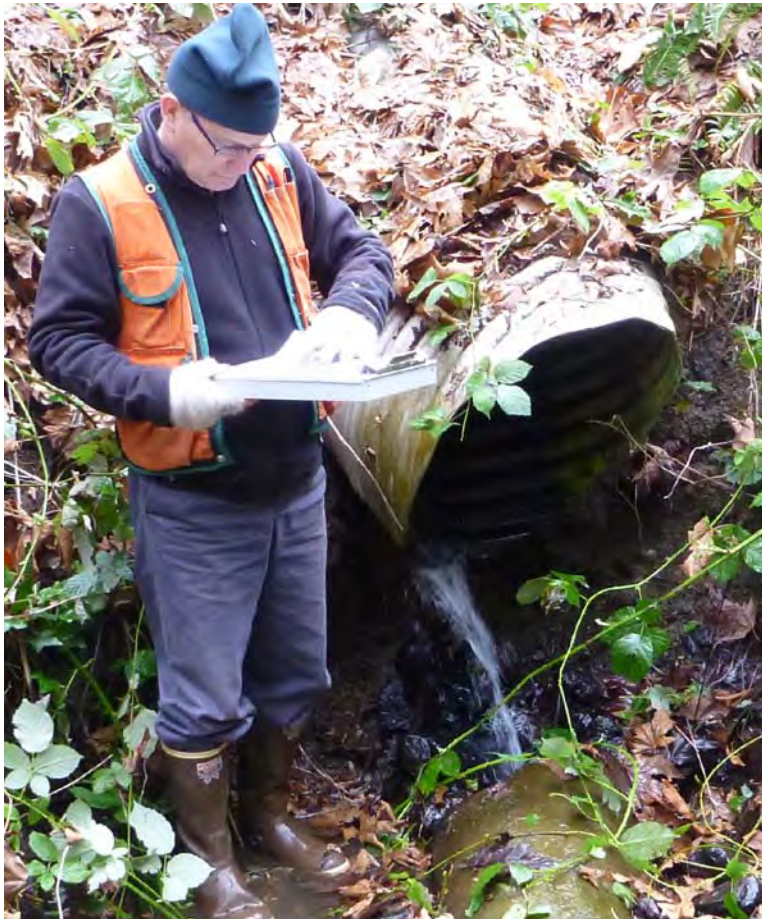
Erosion at Pipe Outlet, same location as above 03/09/2012
