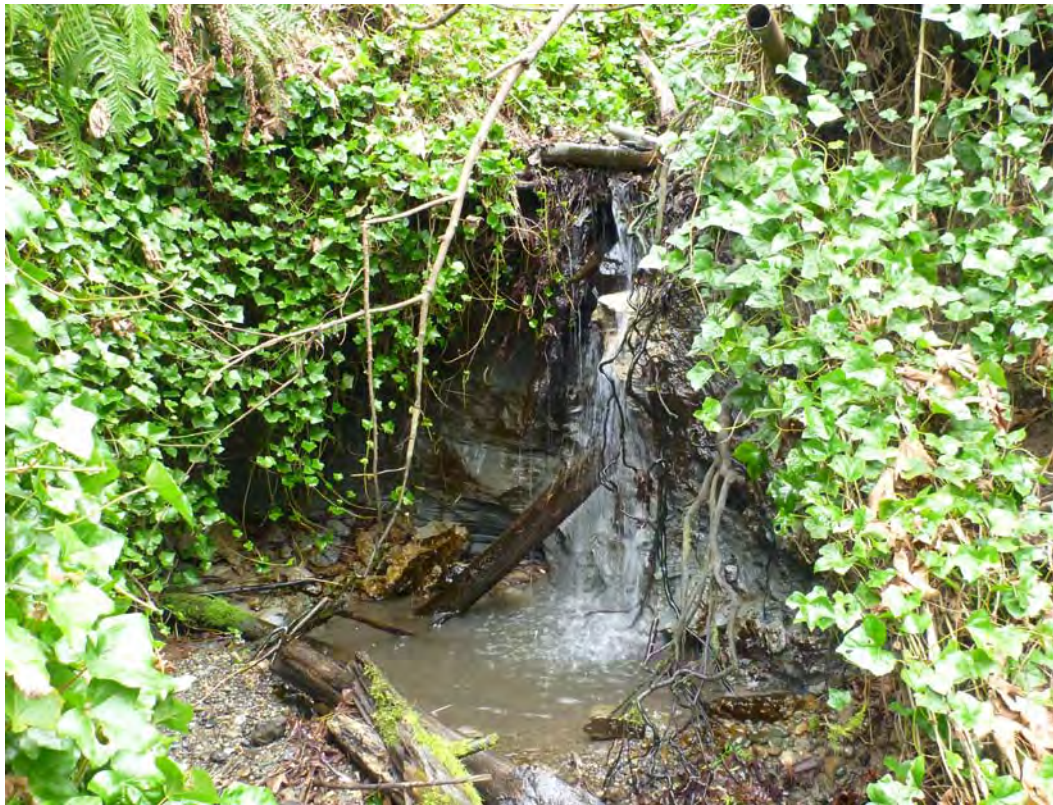
Headcut at Station 2+00 with 10 Foot Drop 3/9/2012
