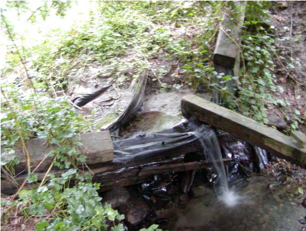
Looking Upstream at Failing Timber Dam 9/28/2006
