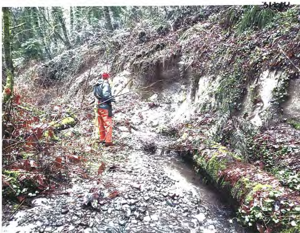
Project 6.5: Eroding bank 31+70 2/15/2011
