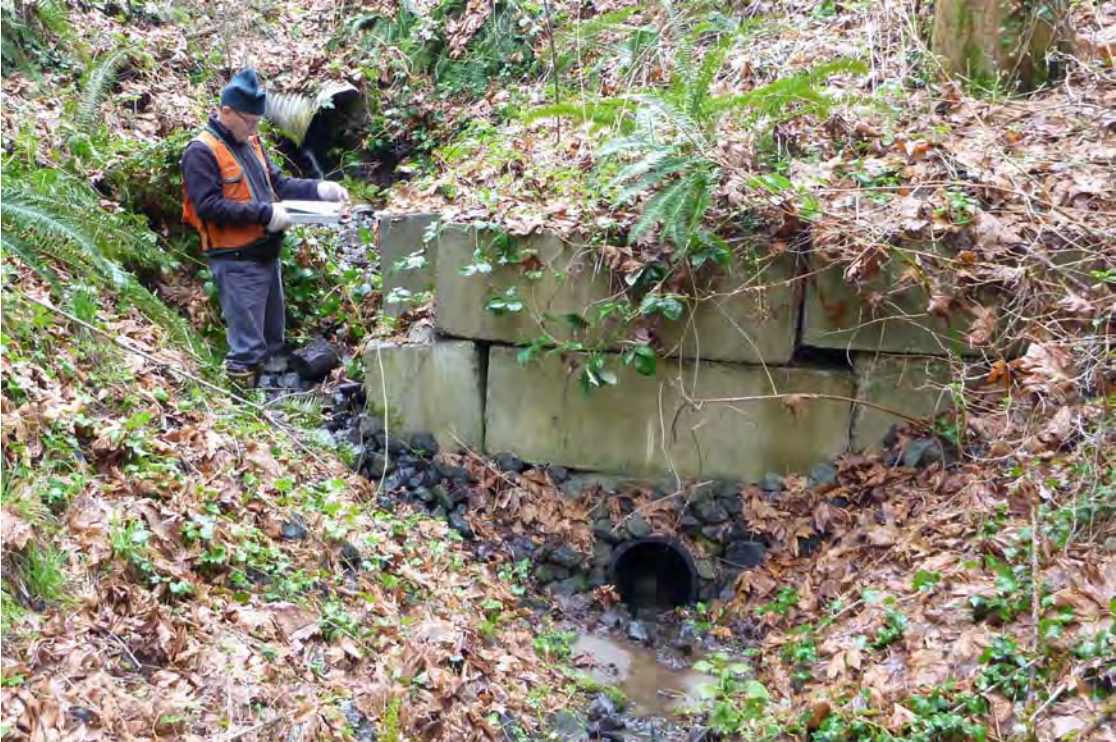
Looking toward East Mercer Way with outfall from road at upper left and culvert draining slope behind camera 03/09/2012
