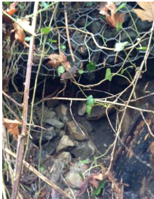
Project 4.2: Failing Gabion Wall 12/22/2011
