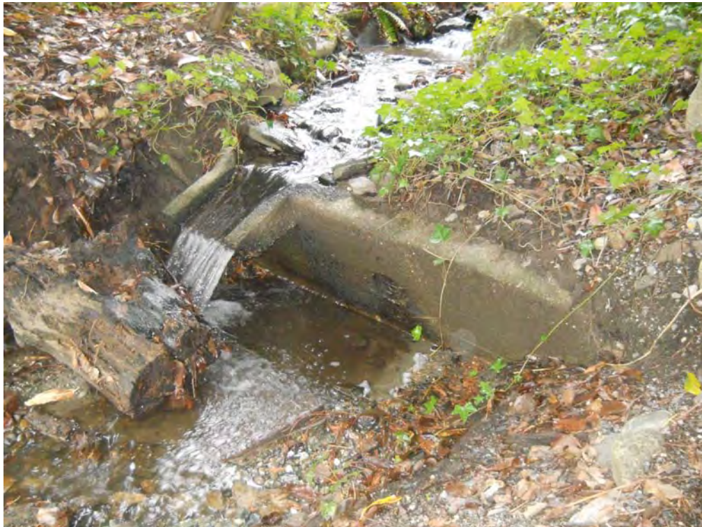
Project 50b.4F: Looking Upstream at Failed Concrete Weir 12/22/2011
