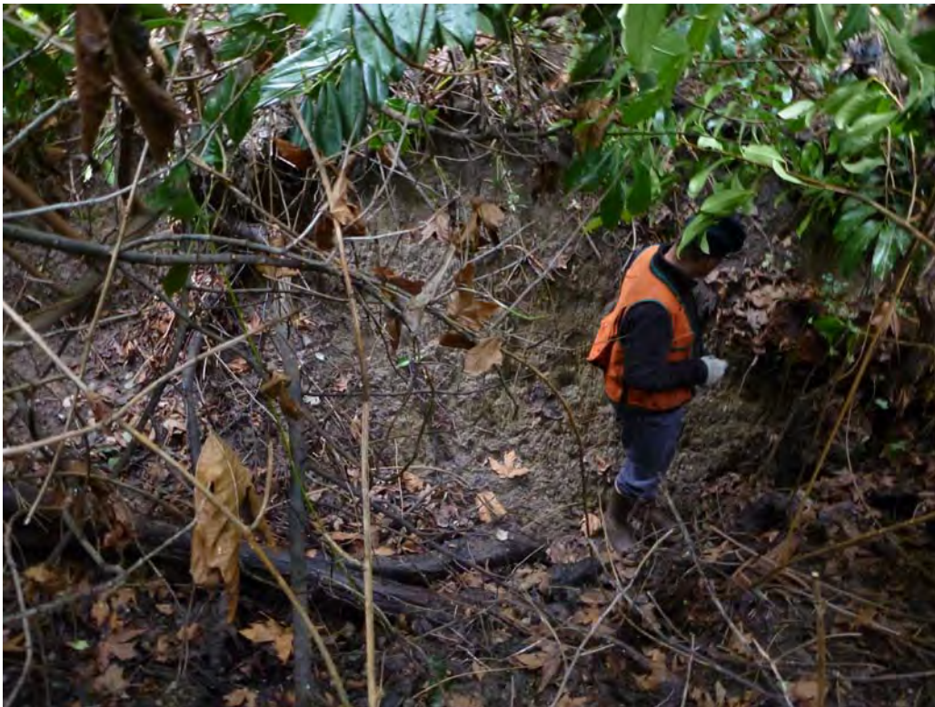
Steep Silty Sand 8' High Banks from Right Bank 3/9/2012
