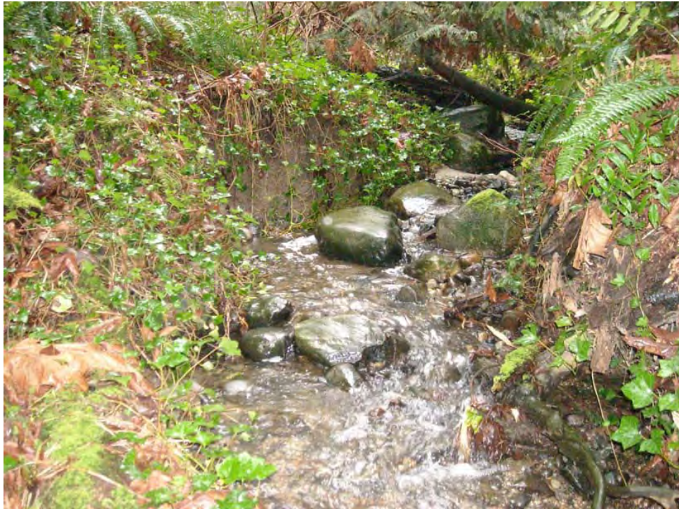
4.3C: Looking Upstream at Bank Erosion at a Stream Bend 3/13/2008
