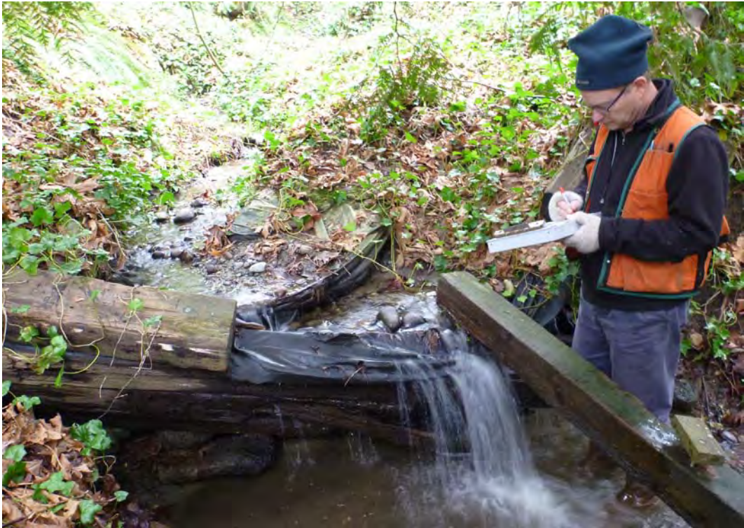
Looking Upstream at Failing Timber Dam 3/9/2012
