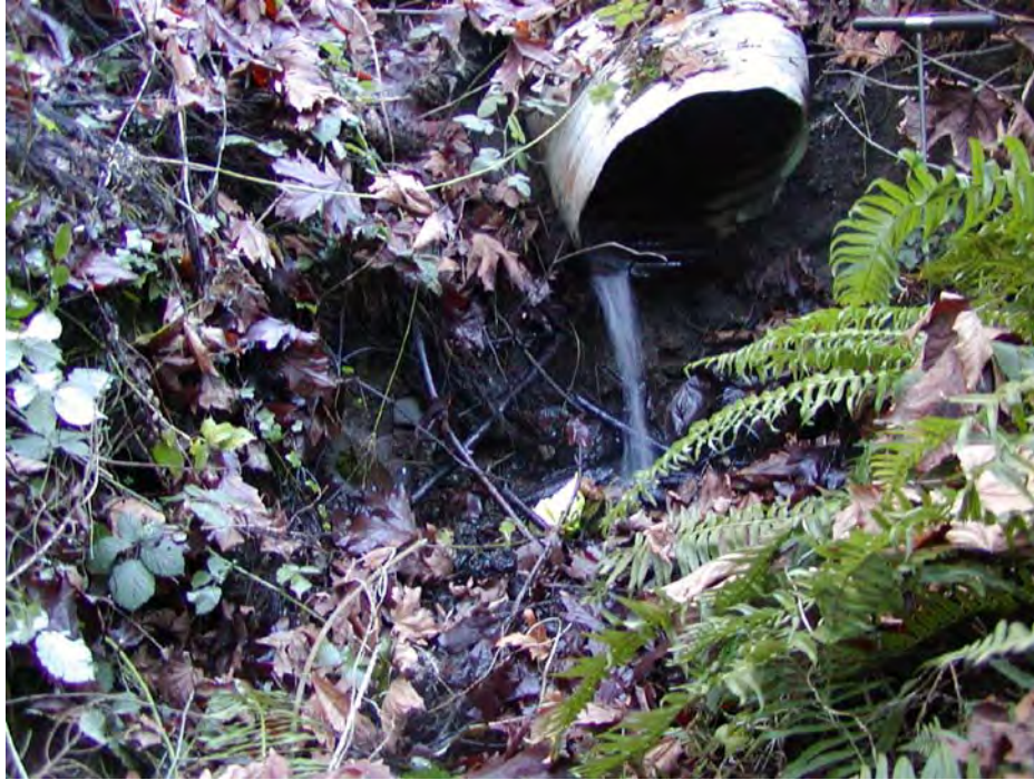
Erosion at Pipe Outlet (pipe crushed) 12/8/2005
