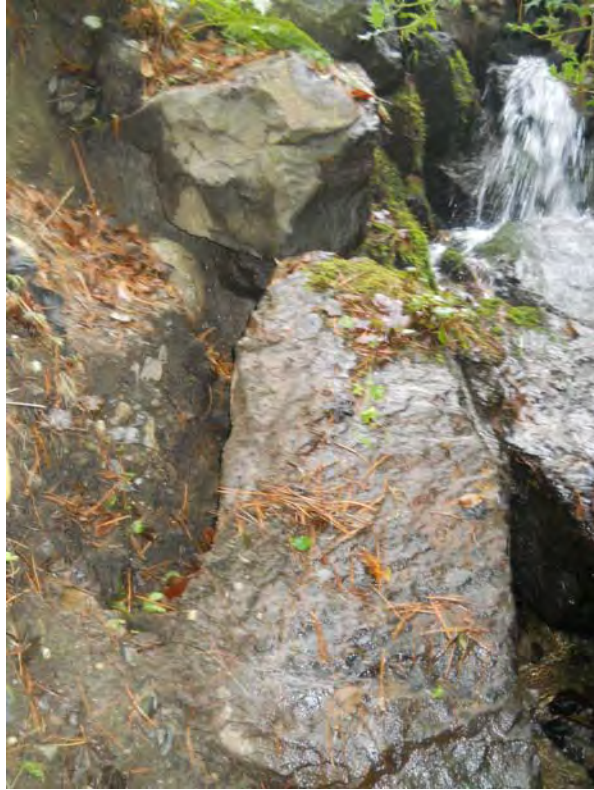
Project 50b.4E: Looking Upstream at Failing Bank Protection at Outlet 12/22/2011
