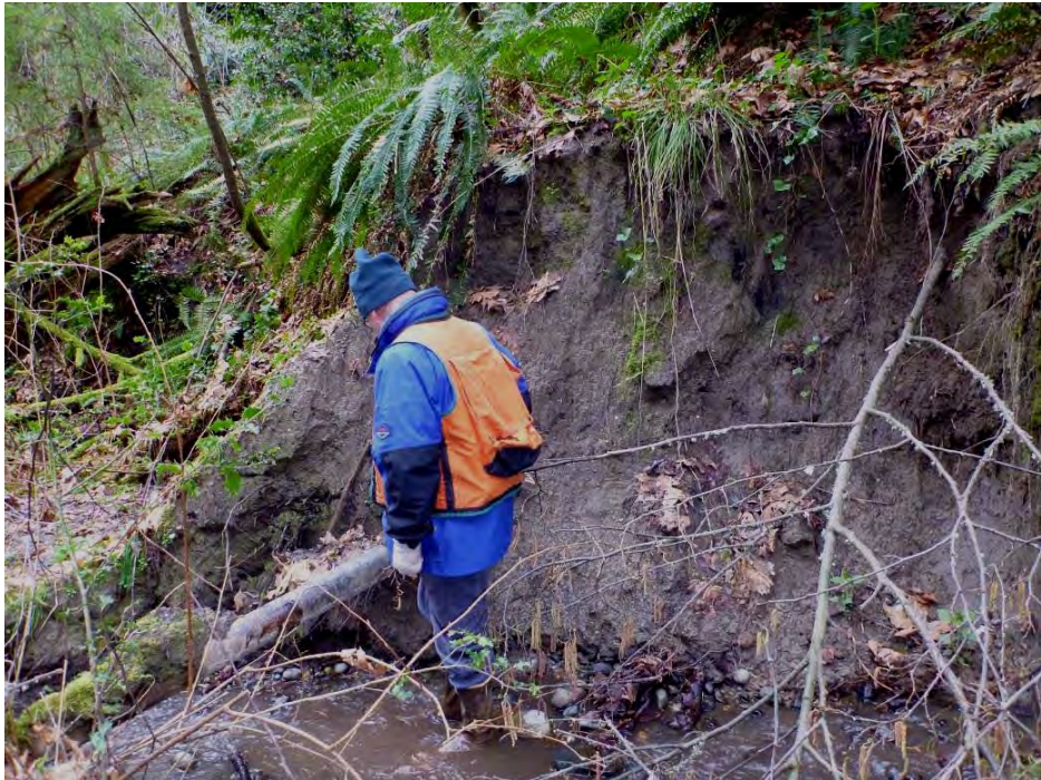
Downstream end of eroding right bank, 7 feet high and 50 feet long, with undercut and separated pipe directly in front of engineer 03/09/2012.
